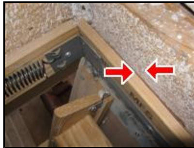
D. Picture 2 Shimming needed
