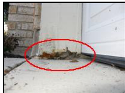
E. Picture 14 Bottom edge of garage door, left side
