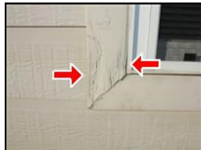
E. Picture 16 Rear window beside chimney
