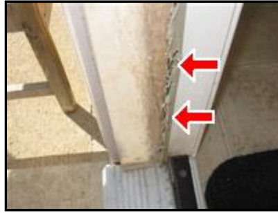
G. Picture 1 Damaged weatherstripping
