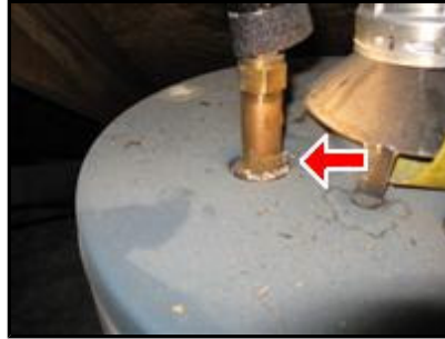
C. Picture 1 Minor corrosion
