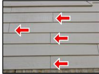
E. Picture 4 Siding gaps on right side
