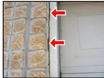
E. Picture 21 Gap between brickwork
