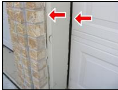
E. Picture 20 Damage to garage door trim
