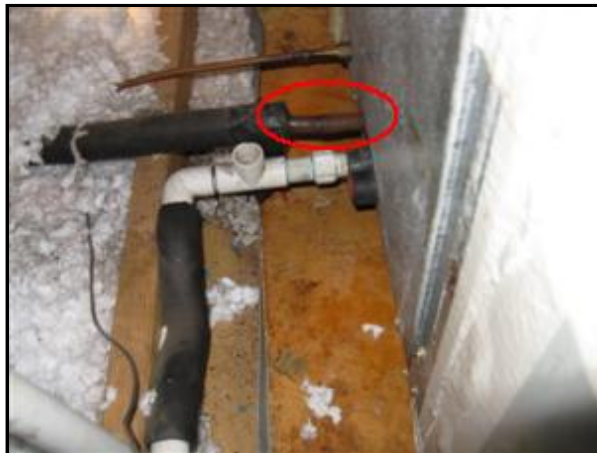
B. Picture 1 Upstairs a/c unit
