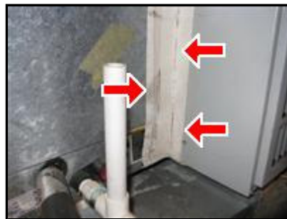
C. Picture 1 Air leaks
