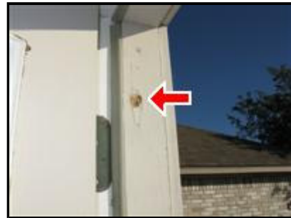
E. Picture 10 Back door trim damage needs sealing
