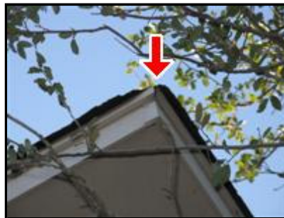
C. Picture 5 Left front corner damage
