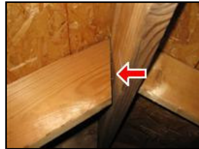
D. Picture 4 Left front rafter gap
